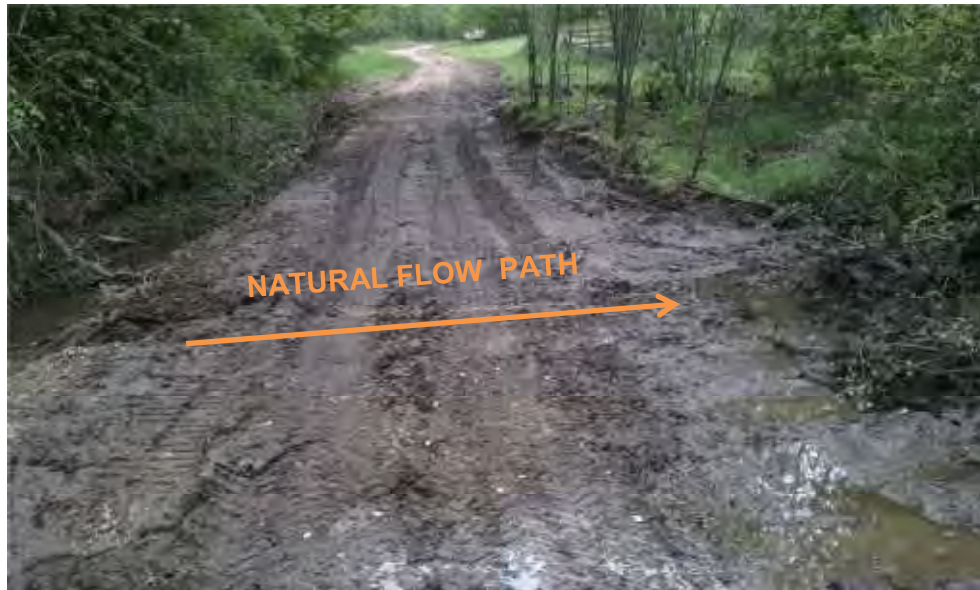
Figure 6. Access road is routinely re-graded which stirs up sediment due to dirt / gravel surface; damage is due to seasonal cross drainage (Photo: HR Green)
