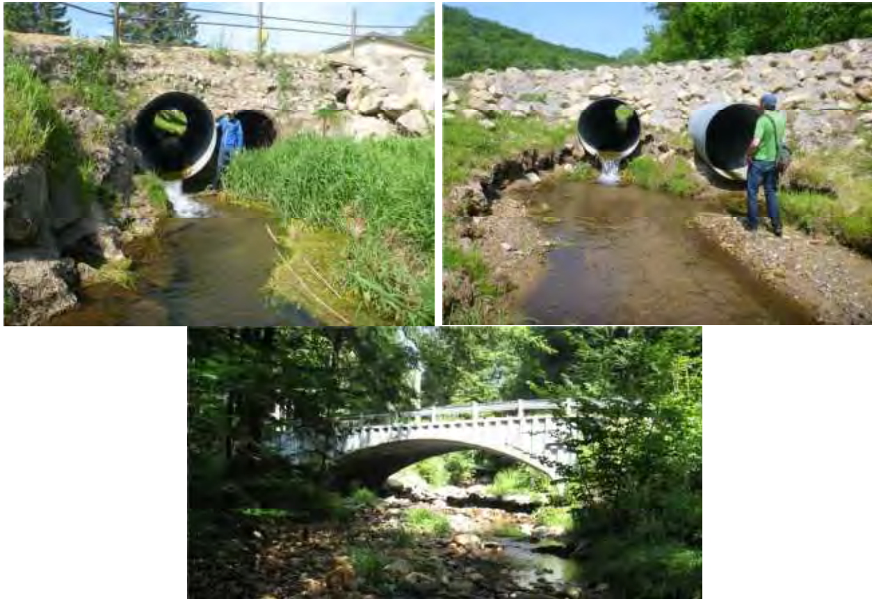
Figure 21. The culverts under both road crossings near the Afton Alps lodge are all perched and undersized, leading to erosion and ecological concerns (top photos). These can be replaced by bottomless arch culverts (left) or bridge spans for better stream flow. (Photos: Inter-Fluve)
