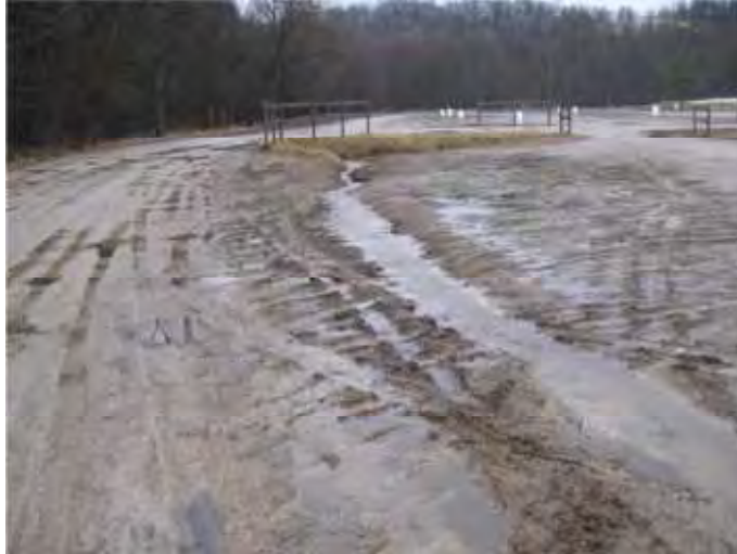
Figure 1. Lower Parking Lot and Road During Runoff Event (Photo: HR Green)
