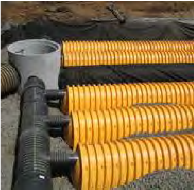
Filtration and storage chamber BMPs with an isolator row of chambers for TSS capture (image StormChamber)
